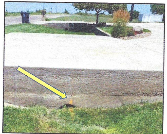
The drainage culvert has become blocked.
